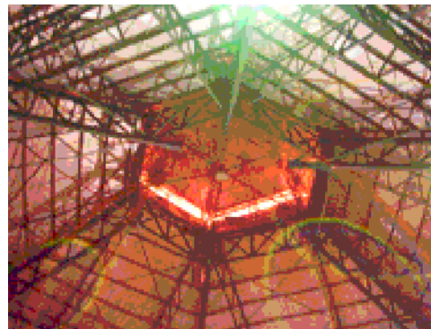
Figure 5: Steel Roof Trusses on Conc. Column Figure 6: Roof Trusses of Cone and Roof Light
